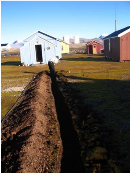
Figure 8.8. Digging by hand. Ditch for power cable to Veteranhytta summer 2005. Photo: Linda Bakken
