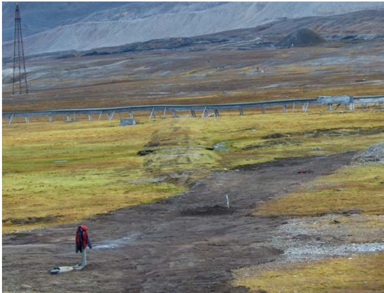
Figure 6.4. Just after closure of a ditch dug for repair of pipelines south of Mellageret, August 2005. Photo: Gunnar Sander.
