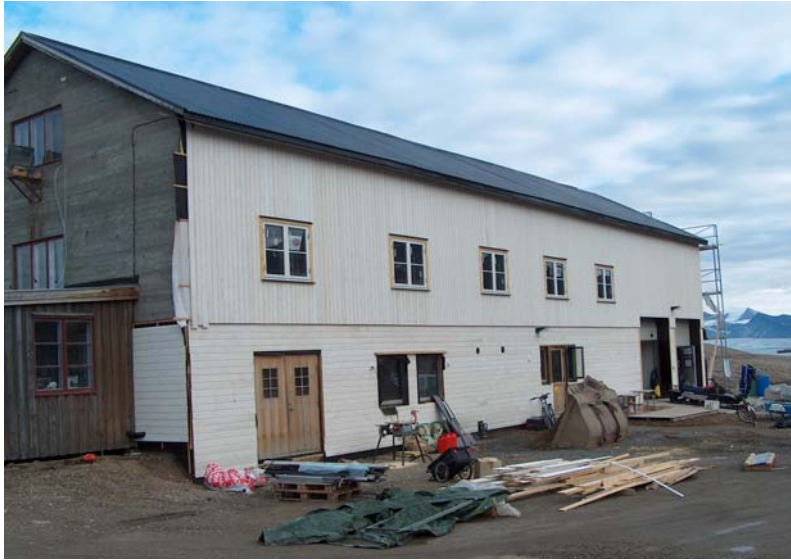
Figure 9.1. Energy saving should be a main energy strategy for Ny-Ålesund. Here “Snekkasjen” is insulated summer 2005. Photo: Gunnar Sander.
