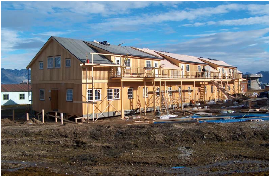
Figure 7.1. Even upgrading of existing houses lead to some wear and tear of the surrounding tundra. Here from Evenstad, August 2005. Photo: Gunnar Sander.
