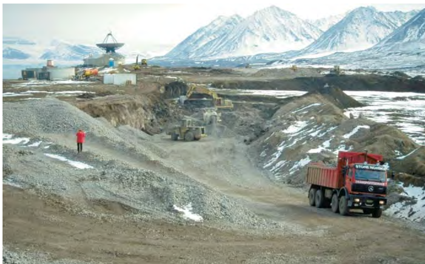
Heavy vehicles working on the expansion of the airstrip at Ny-Ålesund in 1997. Photo: B. Frantzen (NP)
