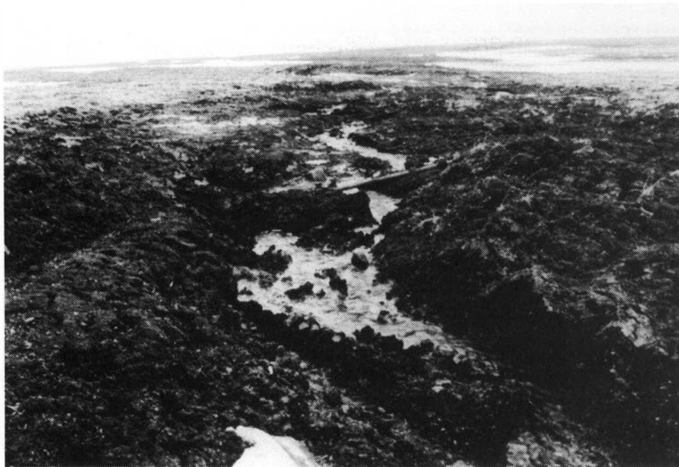
Fig. 16: Track with continuing erosion, type 1A, between Colesdalen and Kolberget.
