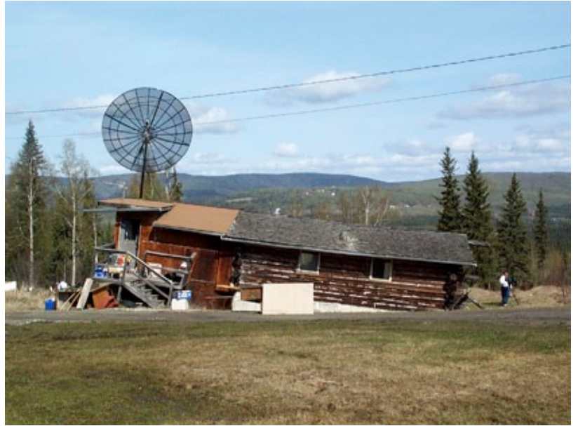
A house affected by melting ice in degrading permafrost. Fairbanks, Alaska, USA, 2004.
