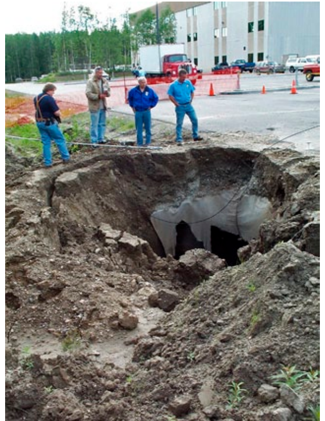
Collapse caused by thawing permafrost. Fairbanks, Alaska, USA, 2009.
