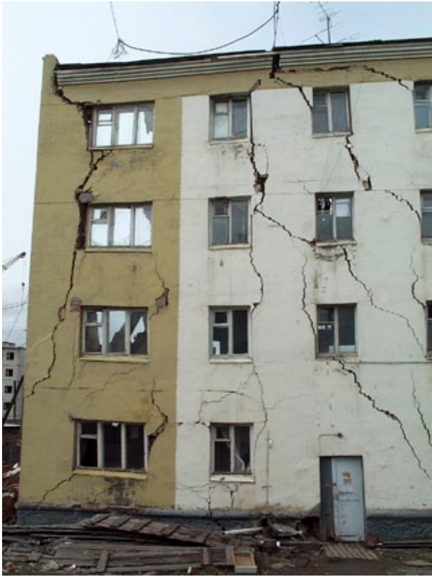
Permafrost thawing has destroyed a four-storey apartment building in Yakutia, Russia, 2001. All photos: Vladimir Romanovsky
