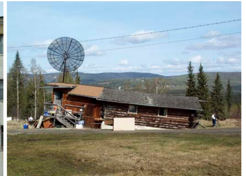
A house affected by melting ice in degrading permafrost. Fairbanks, Alaska, USA, 2004.
