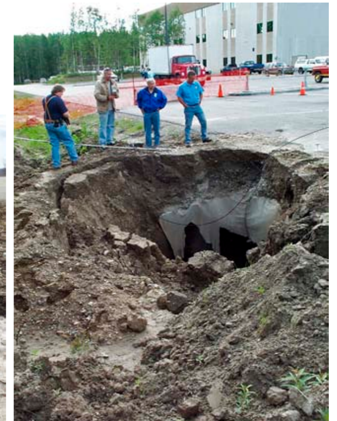
Collapse caused by thawing permafrost. Fairbanks, Alaska, USA, 2009.
