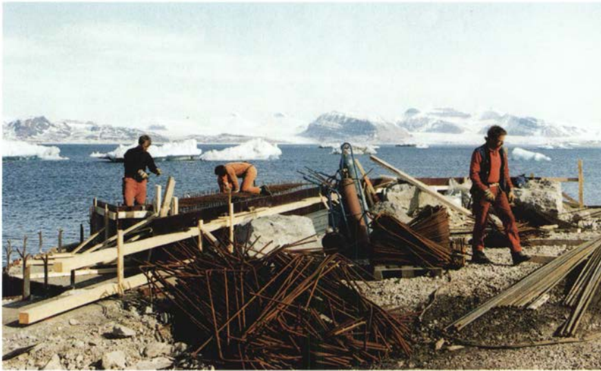
Fig. 97. The new quay in Ny-Ålesund was built as a fortress of heavily reinforced concrete, to make it resistant against attacks from drifting icebergs in the fjord. (V.H.)
