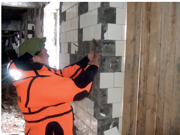
Sampling for PCB in mortar and tile adhesive in Grumantbyen. Photo: Qno Lundkvist, Climate and Pollution Directorate
