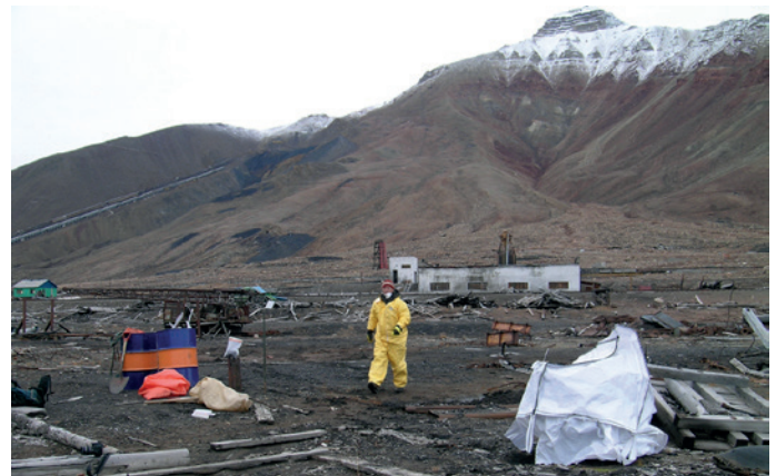
Removal and destruction of high-voltage electrical equipment which leaks PCB in Pyramiden. Photo: Halvard R. Pedersen, Sysselmannen på Svalbard (Governor of Svalbard)
