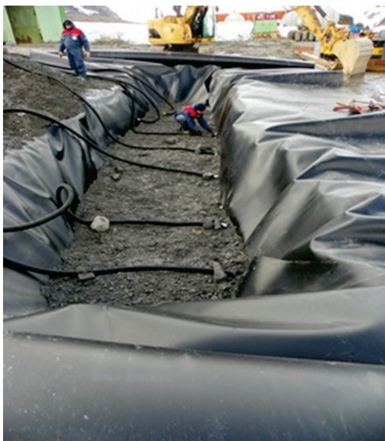
Figure 16. The Brazilian Research Station, Antarctica. Installation of a bioventing system during in situ remediation of diesel-contaminated soil using “biocava” techniques (ATCMXXXIX-CEP6, 2016).
