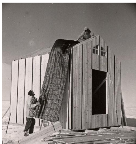
The Rawin Hut is being built during the Maudheim Expedition. Photo: V. Schytt, 1950. Norwegian Polar Institute's Photo Archives.
