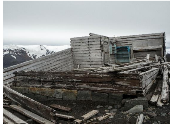
The timber magistrate house in Whalers Bay was built by Norwegians. Photo: Ann Kristin Balto, Norwegian Polar Institute, 2016.
