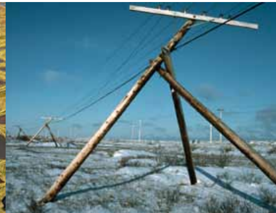
Telephone poles set in tripods for support in the permafrost region of Churchill, Manitoba, Canada.
